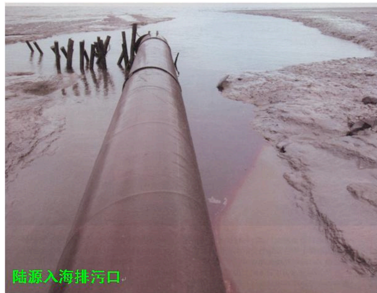
Seaside sewage outfall
